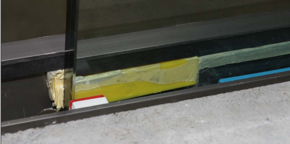
Picture 5: glazing blocks were taped together and introduced at the edges of the glass in the profile (left edge)
