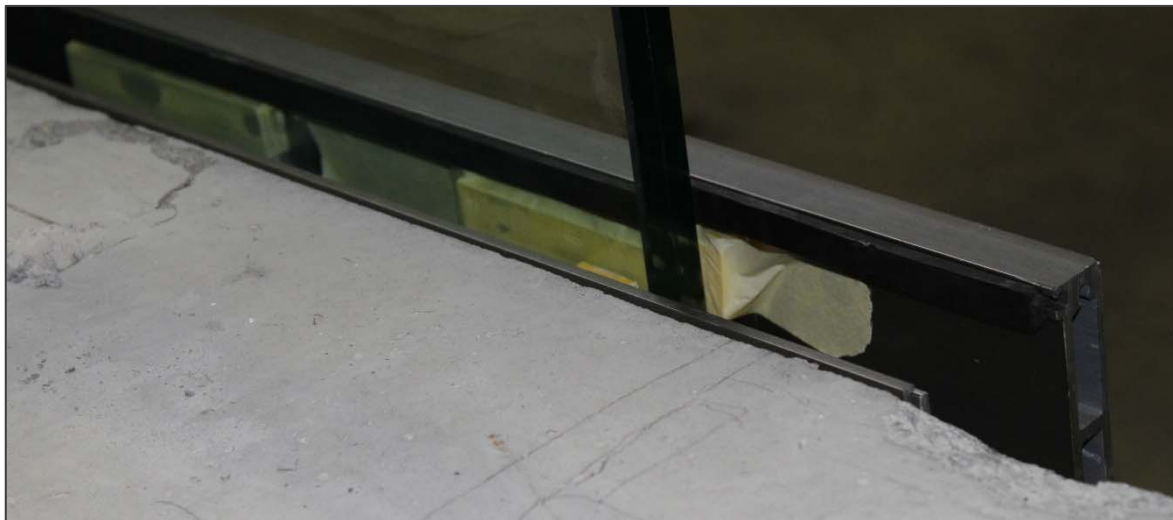
Picture 6: glazing blocks were taped together and introduced at the edges of the glass in the profile (right edge 1/2)
